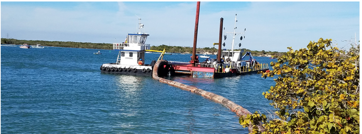
Sedimentation from dredging, pictured here, and other coastal construction, pose major threats to essential fish habitats.
